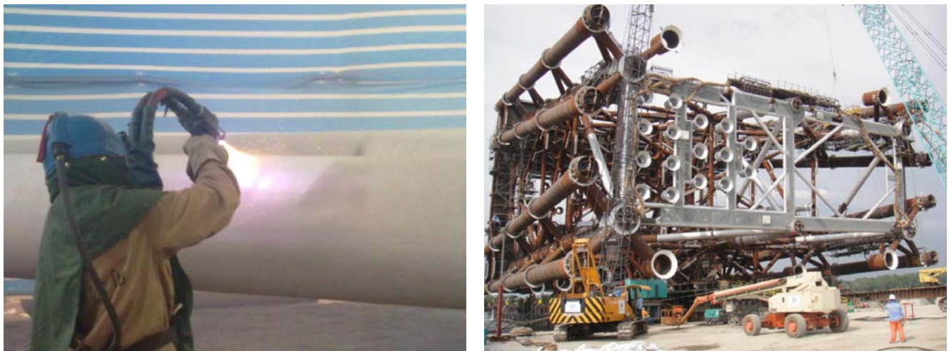
Fig. 6 — From left to right, TSAC application on actual job and completed job.
